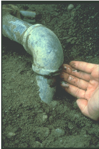
Leaking pipe from UST
